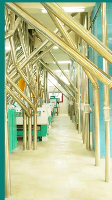
Pipe and cyclone in milling section where contact with product is stainless steel
